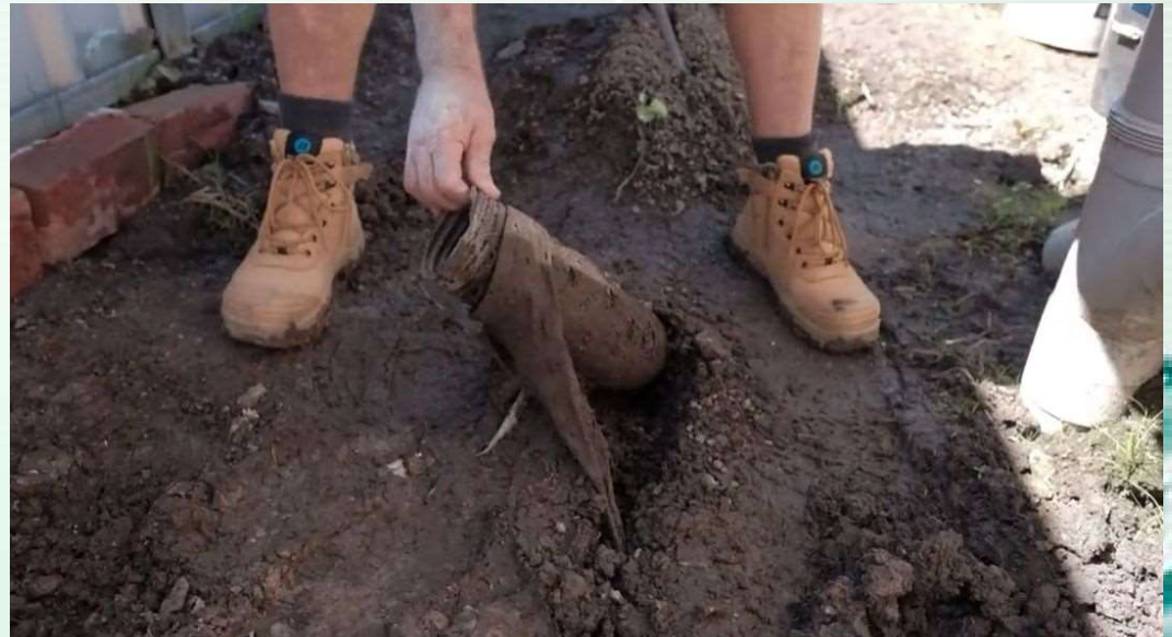
Geotech fabric also becomes blocked
